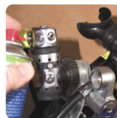
Checks gas and compressed air valves
